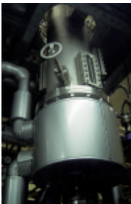
Crystallizer pilot plant
