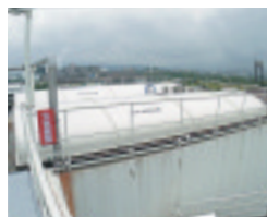
Anaerobic wastewater processing system
