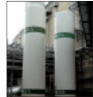
CO 2 storage tank
