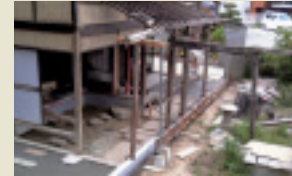
Artists and local residents of the island cooperate in refurbishing run-down vacant houses. Such creation of a space for displaying work is also a part of our art project.
