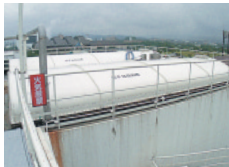
Anaerobic water processing system
