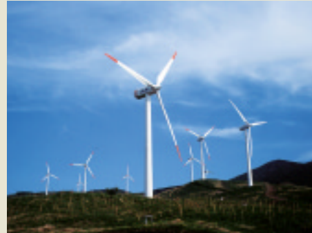
Wind-powered generation facilities
